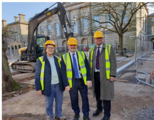
Council Leader, Patrick Farrington, Councillor Mrs. Frances Beatty, Cabinet Member for Economic Development and Planning in Market Square overseeing the laying of kerbing
