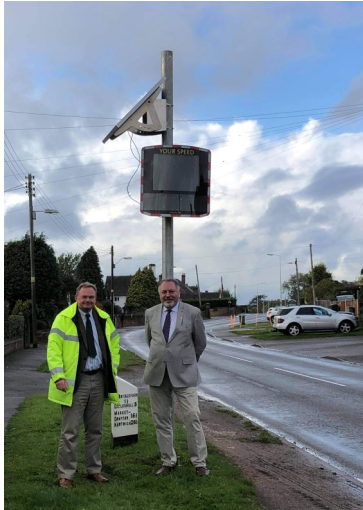
At the installation of the latest Speed Indication Device, with Councillor Ray Sutherland from Creswell Parish Council—October 2020
